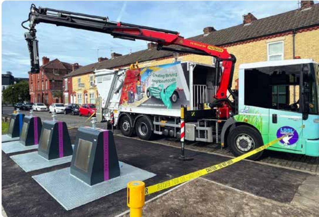
LCC underground bin collections which free up space within the building and help prevent odours and mess
